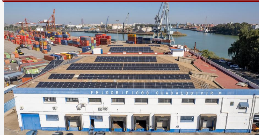
Portofrio Logistic 239,76 KWp/444 modules 2023
