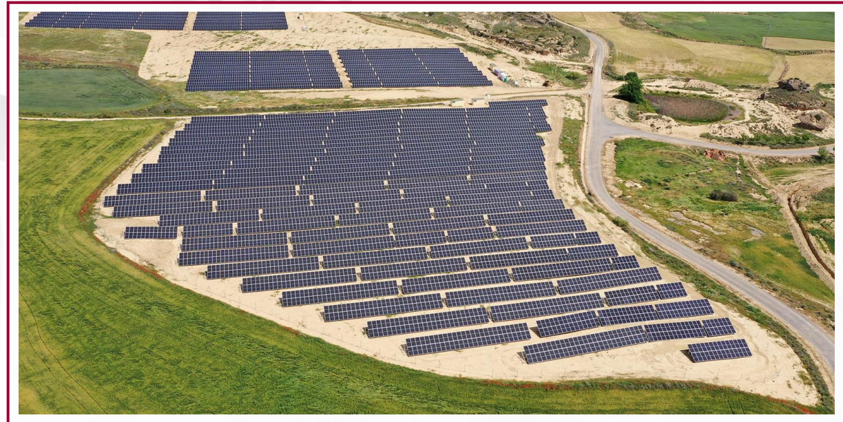
Tormillo III y IV photovoltaic generation plant in Huesca 2.4 MW capacity 5.2 K modular solar panels
